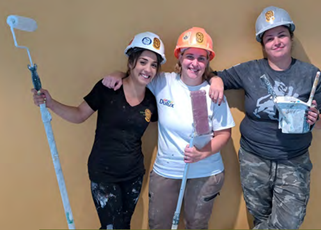
DC 46/LU 557 (Toronto) painters working on the big addition to the Peel Manor Long Term Care Centre in Brampton. L to R: Andreia Ganhadeiro, Lynn Mioducki, and Diana Andrade.
